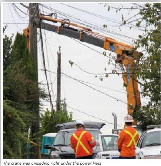
The crane was unloading right under the power lines
